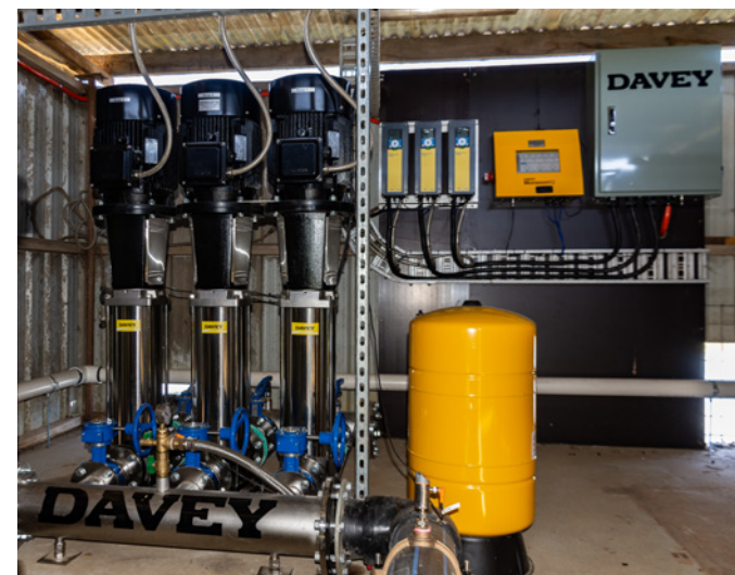
Top Rob gets familiar with the Davey Monsoon IQ interface Bottom The system installed at De Bortoli
